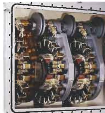
Waukesha UZD Load Tap Changer
