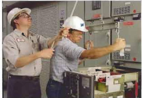
Trained WES Service personnel can perform breaker service in our shop or at your location. Service work at your location can be with your tools and procedures, or ours, depending on your needs.
